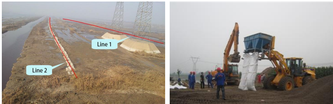
Fig. 9. Gangqing dual pipeline before submerged and local scene of emergency maintenance operations
