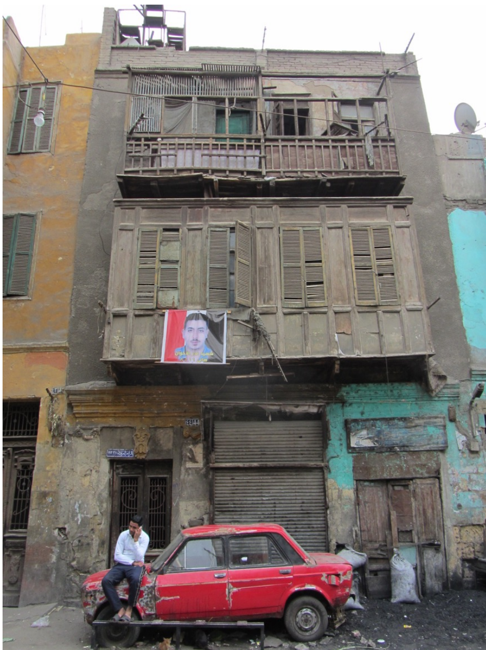
Figure 13: A mixture of European and local influences in Maspero. The wooden box balcony is a typical architectural element in medieval Egypt. The porch and the keystone are Western. The poster in the balcony reads "Hany, martyr of the Muslim Brotherhood treason" 2013. C: author.
