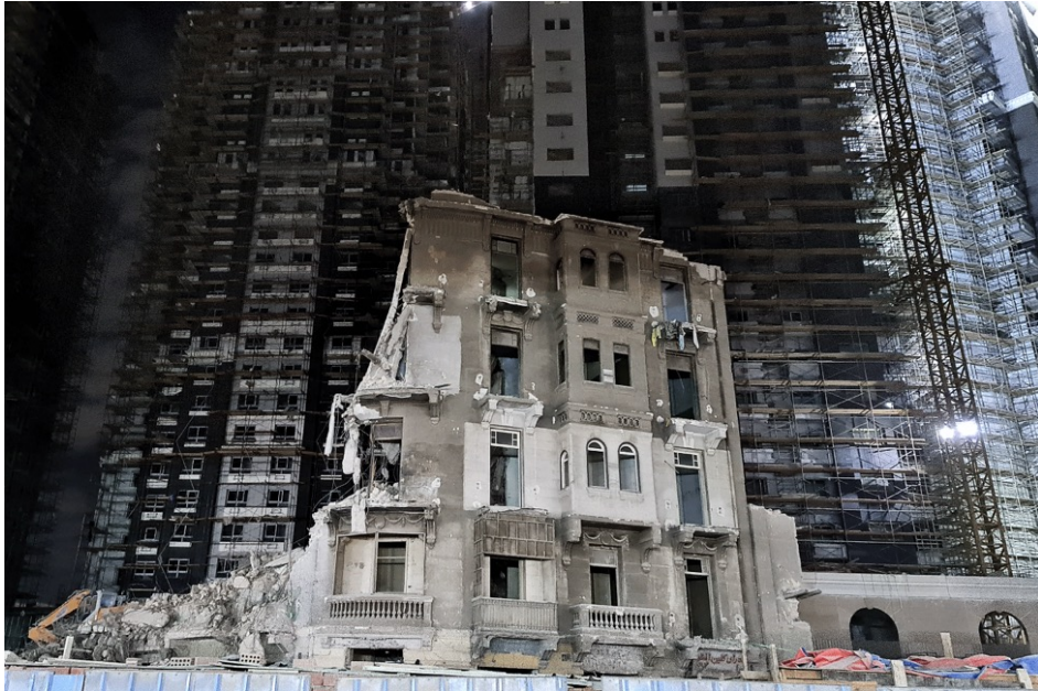
Figure 32: The Maspero towers rising over the city. The beginning of demolishing the listed buildings after all. C: Mohamed Hozyen. https://www.mohamedhozyen.com/projects . circa: 2020.
