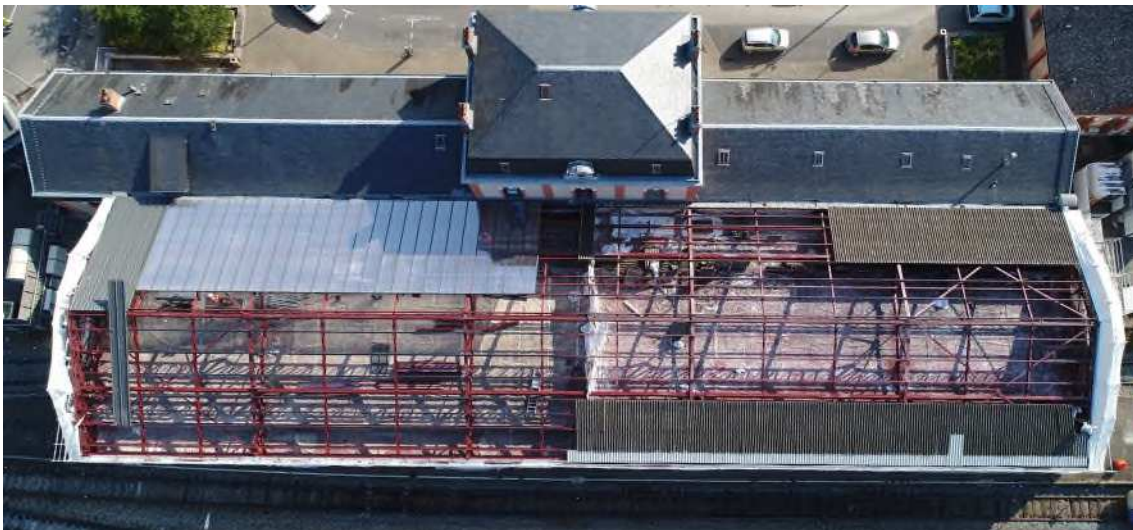
Figure 15 : Example of complete replacement of the roofing: aerial view of the restoration of the shed of the Gare de Tulle in 2019, Tulle, France (Picture from SNCF). Right side: old fibre cement panels. Left side: new steel decks and polycarbonate panels.
