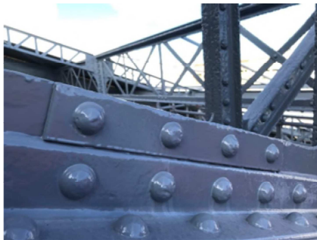
Figure 23: Local repair of a chord with added riveted plates in the train shed of Troyes renovated in 2021, Troyes, France (Picture from SNCF).
