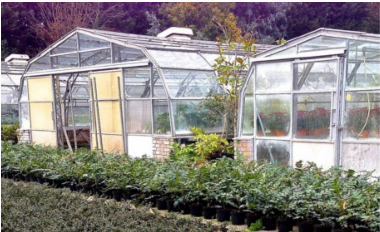
Figure: 25: Wolves Lane Centre has an impressive complex of glasshouses dating from the 1960's but they are expensive to restore and run. Source: OrganicLea.
