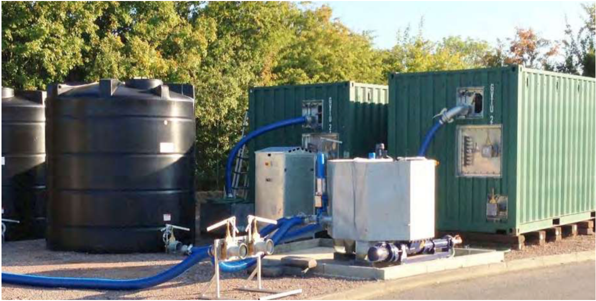
Figure 21. Developing an Anaerobic Digester (image by Tom Dobson, Public Works)
