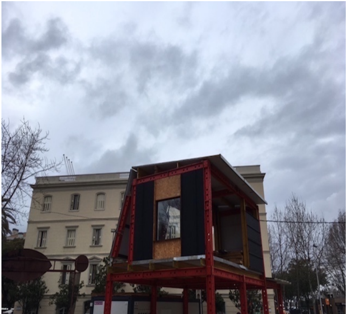
Figure 44. Ateneu for a Community of Squatters, Central Square of Sant Boi, Barcelona
